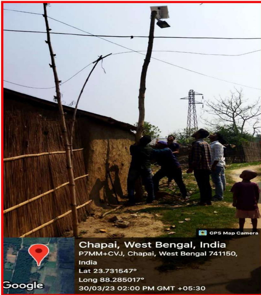
Solar light installation at Chapai village
